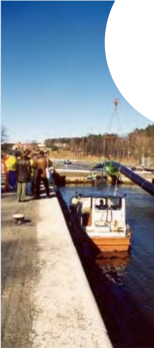
Pulling of Ø 1000 mm PE pipe over a lock in Sdertlje, Sweden, 2000
