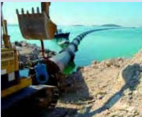
Submerging of the first 1500 m section of a Ø 1200 mm PE pipe sea outfall in Sibenik, Croatia, 2004
