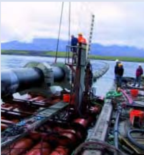
Connection of two ready weighted Ø 1400 mm pipe sections over a pontoon, Iceland, 2001
