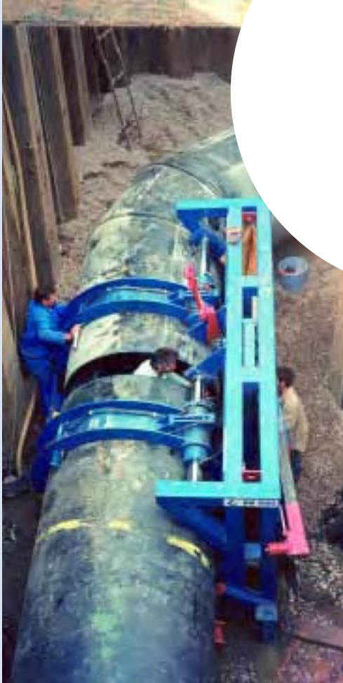
Welding of the on-land pipe section inside the cofferdam, Ø 1600 mm pipe, Antalya, Turkey, 1998
