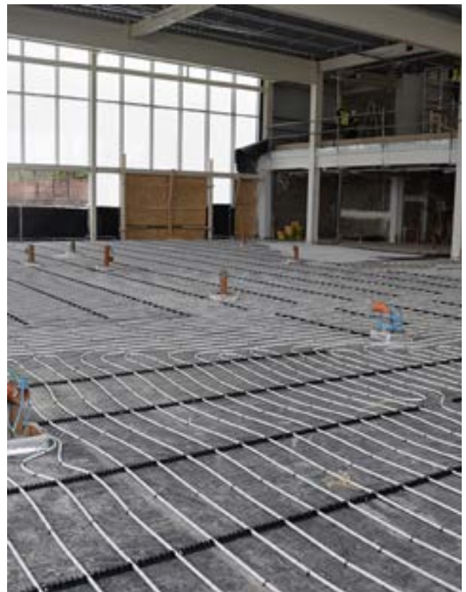
Pipelife Underfloor Heating installation for the Jaguar Car Showroom in Cork, Ireland.
